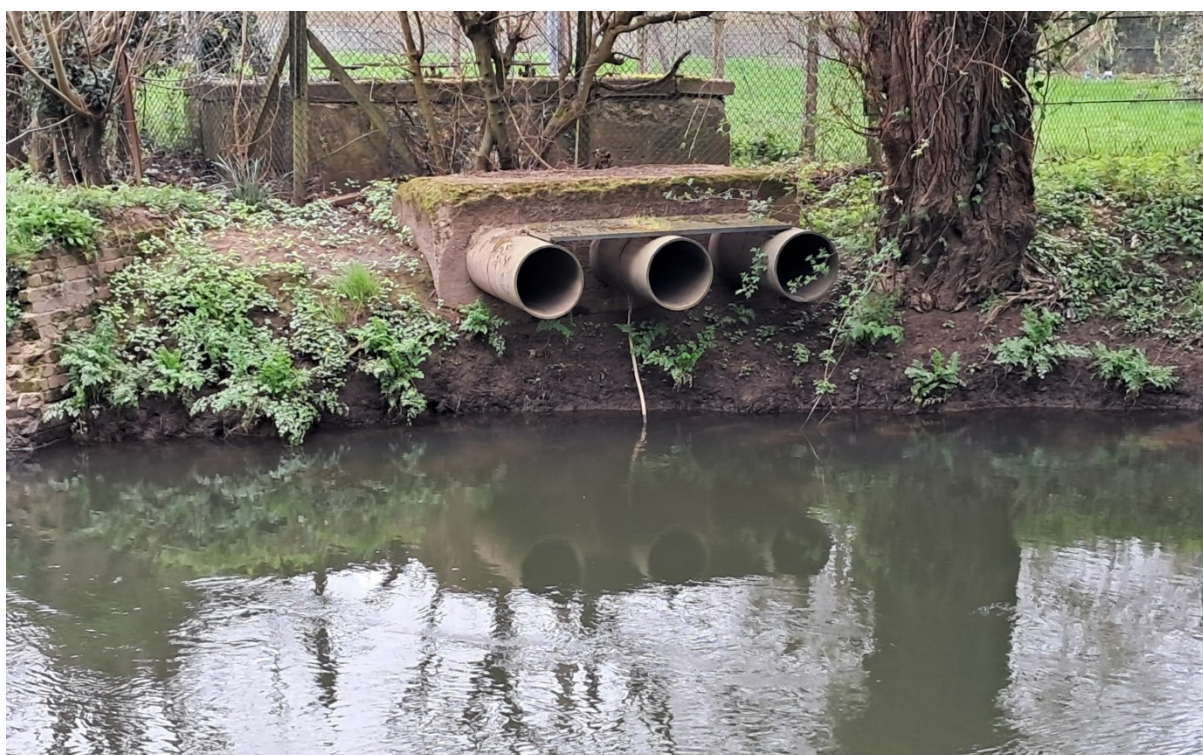
Figure 3 Hoo Brook Pumping Station outfall
